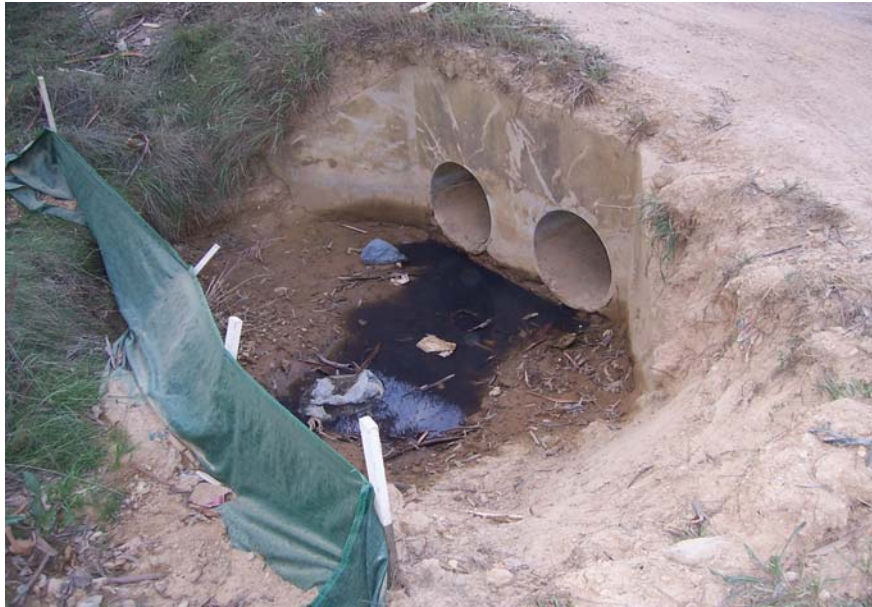
Photo 9: Evidence contaminated surface water discharge to stormwater system flowing under road to adjoining property to North of the site.
