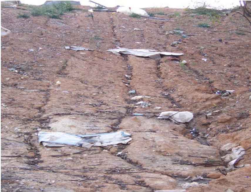
Photo 7: Significant erosion of batter slopes
